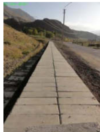
Picture 13. New cable duct between tunnel and switchyard site (Status in October 2019)
