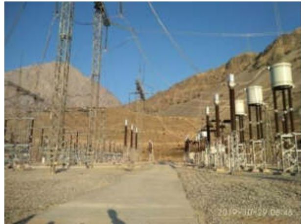
Picture 11. Clean switchyard site, most of works are finalized (Status in October 2019)
