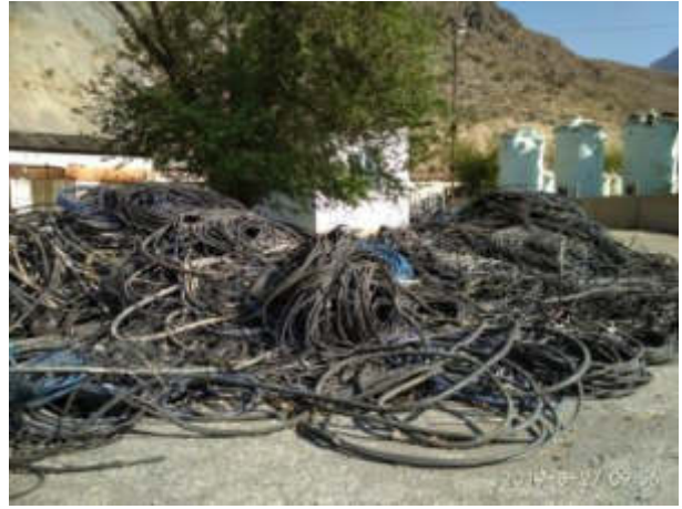
Picture 27. Dismantled cables were removed from site and stored at storage area of Toktogul HPP (Status in August 2019)
