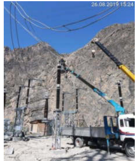
Picture 7. Steeplejack work at 500kV substation of Toktogul HPP (Status in August 2019)
