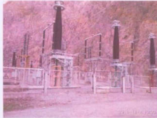
Pic.2. Area of Distribution Point 500 kV of Toktogul HPP
