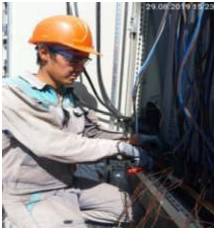
Picture 32. The worker wearing PPE at 500 kV substation of Toktogul HPP (Status in August 2019)
