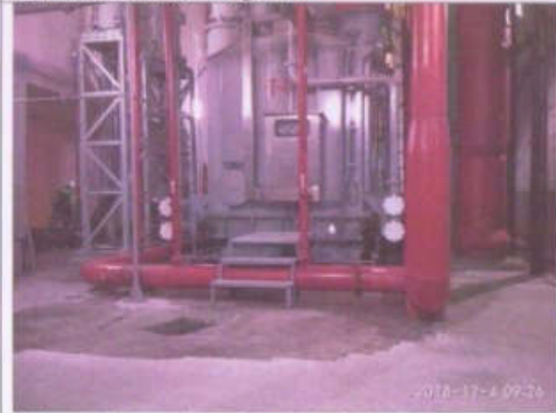
Pic. 3. Area of the main transformer T4 of Toktogul HPP
