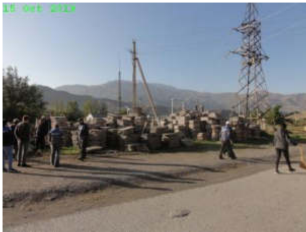
Picture 16. Intermediate storage of old cable duct cover plates (Status in October 2019)
