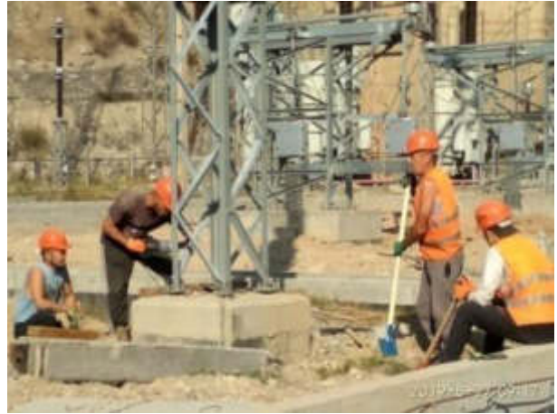
Picture 35. Two workers working without reflective vests (Status in August 2019)
