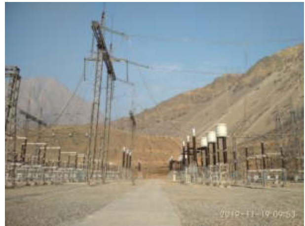
Picture 21. 500 kV substation after rehabilitation works (Status in November 2019)
