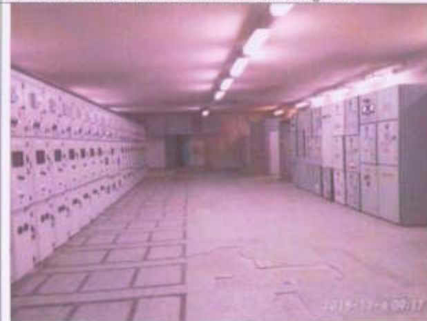
Pic. 4. Area of 6 kV Central Set of Distribution Equipment
