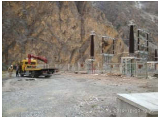
Picture 17. Works on preparation for gravel covering at 500 kV transition point (Status in October)
