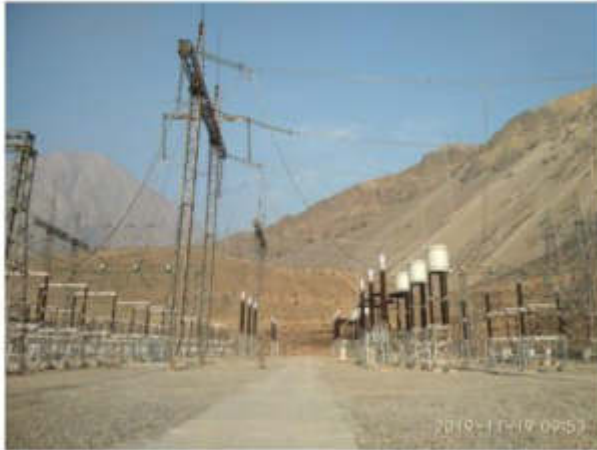
Pic.1. Area of 500 kV Substation of Toktogul HPP (Status in November 2019)
