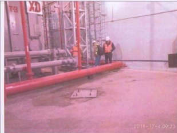
Pic. 2. Area of the main transformer T 3 of Toktogul HPP
