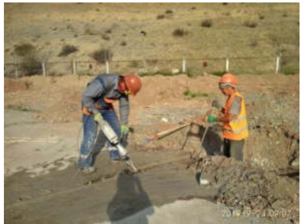
Picture 33. Ear protectors are in used by worker while working with a perforator (Status in September 2019)
