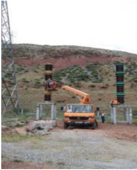
Picture 2. Dismantling works at 500kV substation of Toktogul HPP (Status in July 2019)
